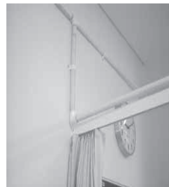
Figure 1. PVC pipe carrying vacuum to the casting station.
