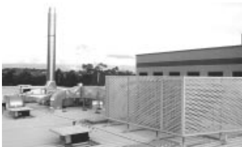
Figure 2. Fan and filter units on roof.
