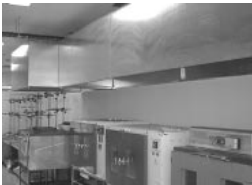
Figure 3. Extraction hoods above ovens.
