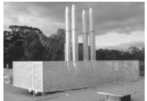
Figure 5. Fans, ducting and exhaust stacks on roof.
